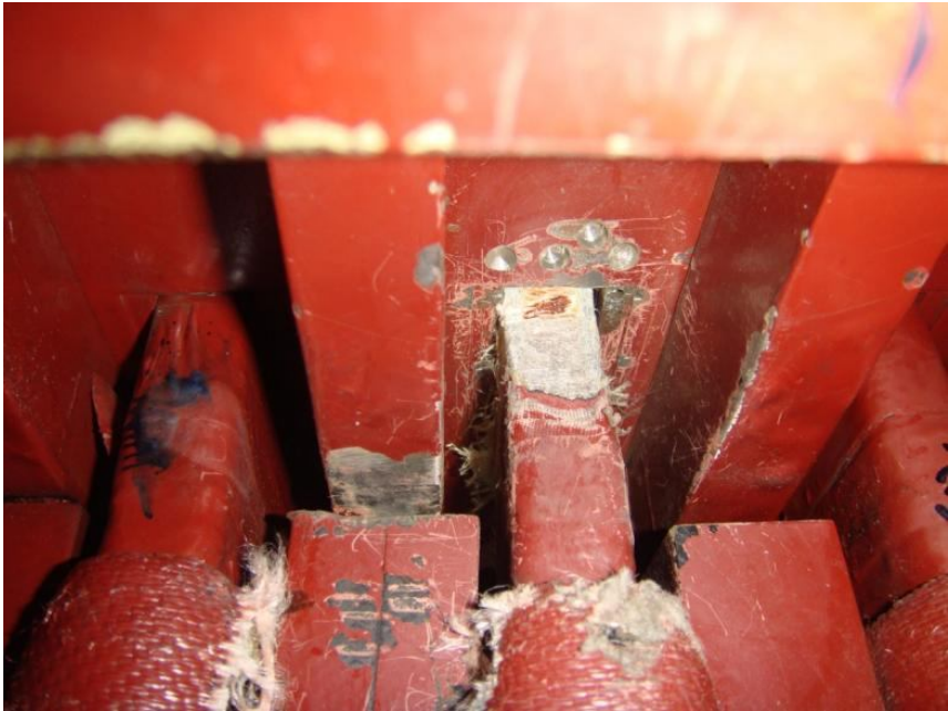
Fig. 3.1 Slot 130 where insulation was removed between conductor and Slot walls for a depth of about 3cm.
