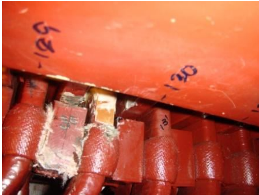
Fig. 3.2 The status of the slot after applying the insulation and slot filling
